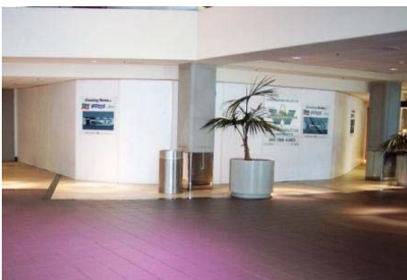
July 2006 - construction has begun on the new restaurant on the lower level of Terminal A at Sacramento International Airport.
